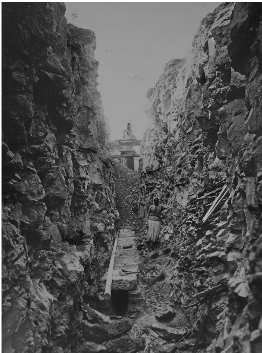
Fig. 4: Construction of a drainage channel, 19th-century photo (courtesy of GMIR Museum, St. Petersburg)
