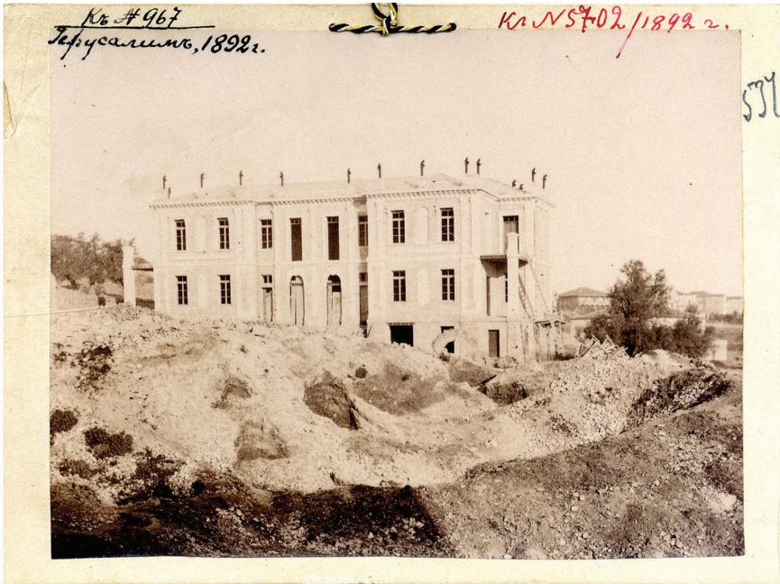
Fig. 6a: Consular House in Jerusalem under construction, 1892 (courtesy of AVPRI State Archive, Moscow)
